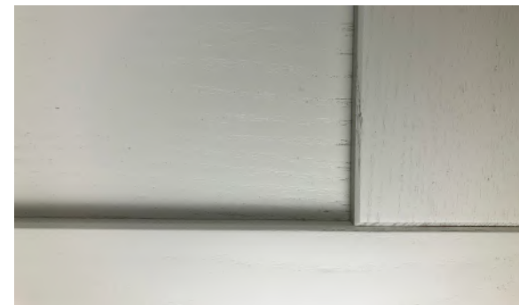
✓ DOOR FRONT CENTRE PANEL PAINT COVERAGE
